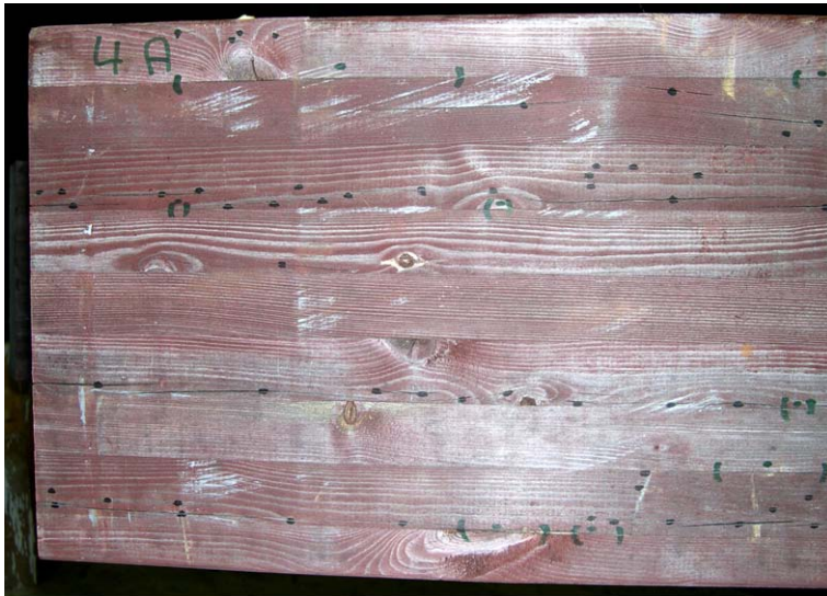
Figure 4.6 Beam 4A. Glue line openings and cracks
